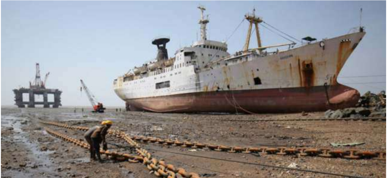
Workers pull a rope tied to a decommissioned oil rig to dismantle it at the Alang yard.
