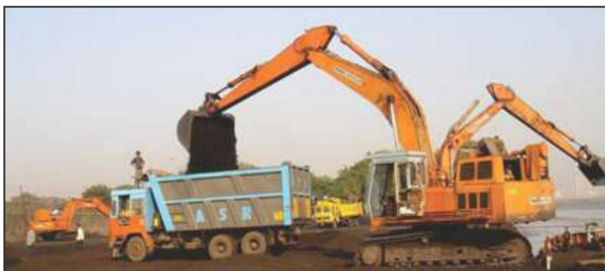
Coal handling with excavators creating dust at Haji Bunder.
